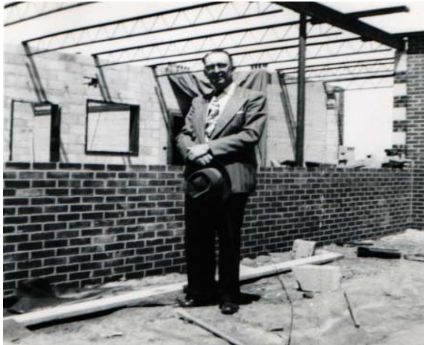
H. E. Pentecost (manager) at the building site of Forked Deer's new office
