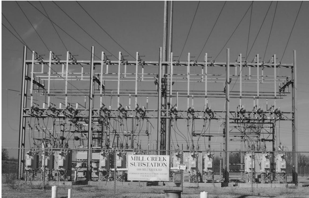
Mill Creek Substation
